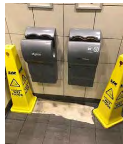
poor solution underneath hand dryers
